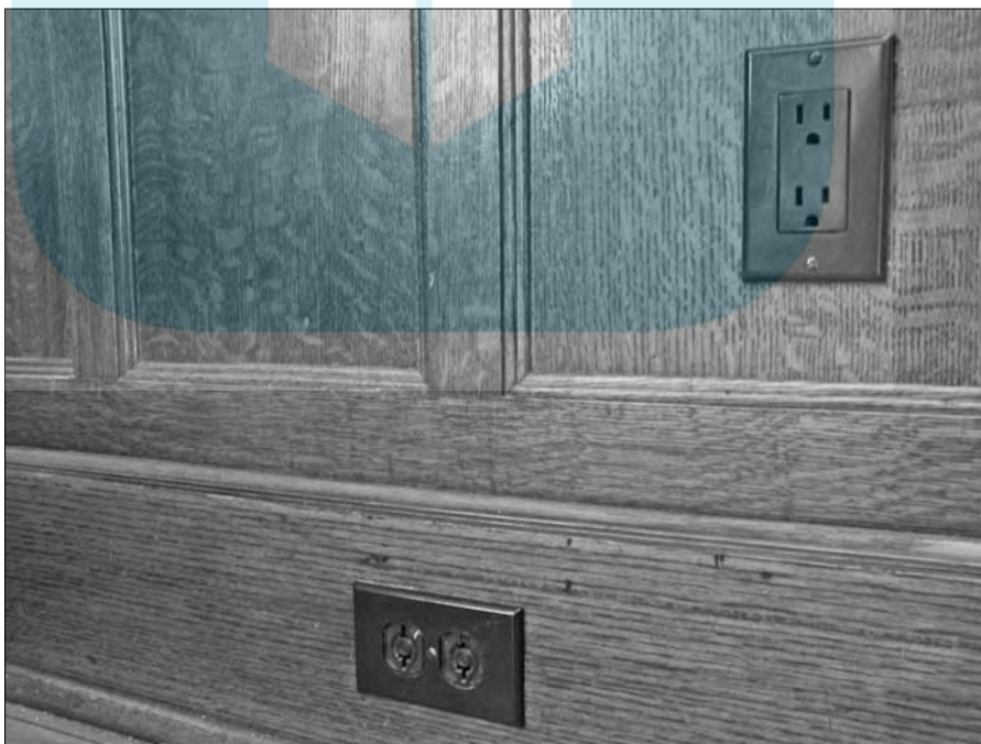
Figure 3-6: The lower baseboard receptacle was originally installed in 1920.
